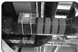
Central AC Plant (PVR Cinema)
